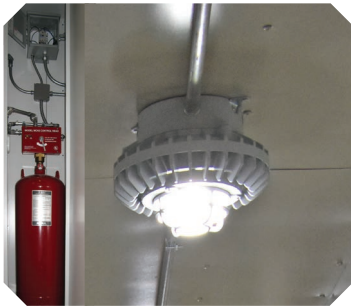
Fire Suppression System
