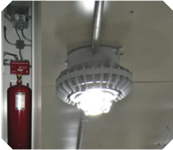
Fire Suppression System
